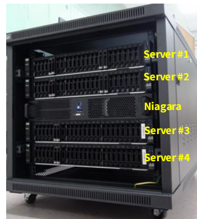
[Rack-Scale System with Niagara]
